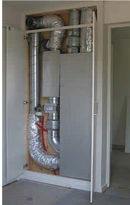
Fig. 2.4.1: Illustration of a heat recovery unit placed in connection to the ventilation system in a closet. This solution makes the maintenance easier.
